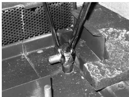
Burner Orifice Removal
